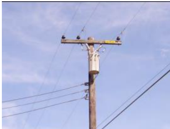
Exhibit 4-13. Single transformer bank
