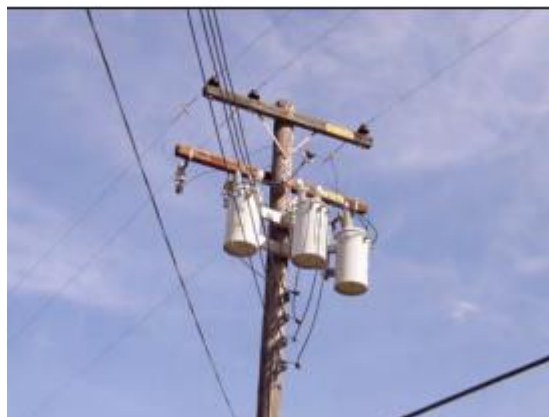
Exhibit 4-15. Triple transformer bank
