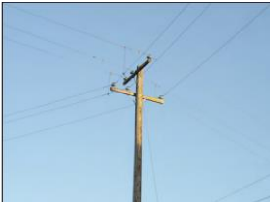
Exhibit 4-12. Double crossarm, three phase corner pole
